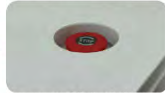
Emergency push button device. In case of emergency, quick power failure
